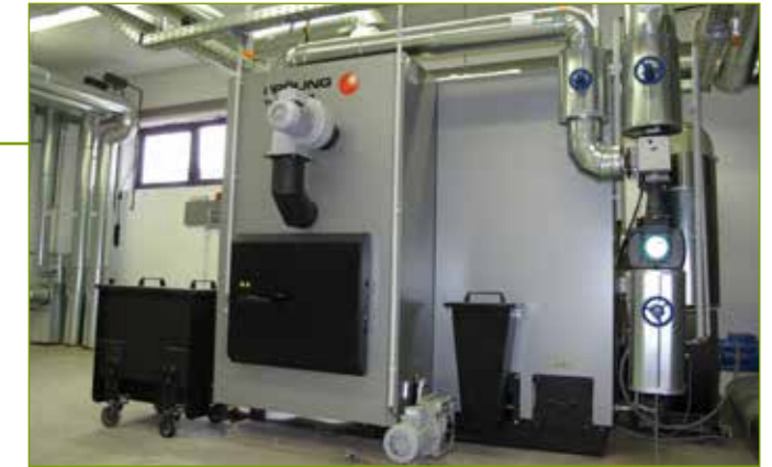
Recent wood chips-heating system (local heat supply)
