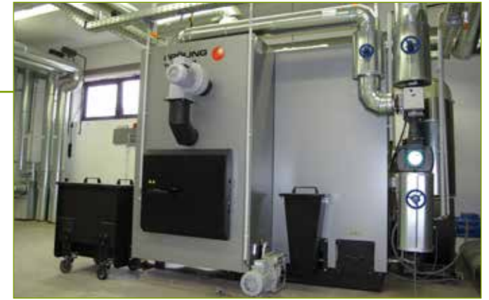
Recent wood chips-heating system (local heat supply)
